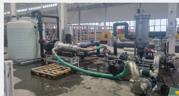
High Voltage Energy Test System(DHP8.2 60Bar + HEX(S)-70/60-3)
