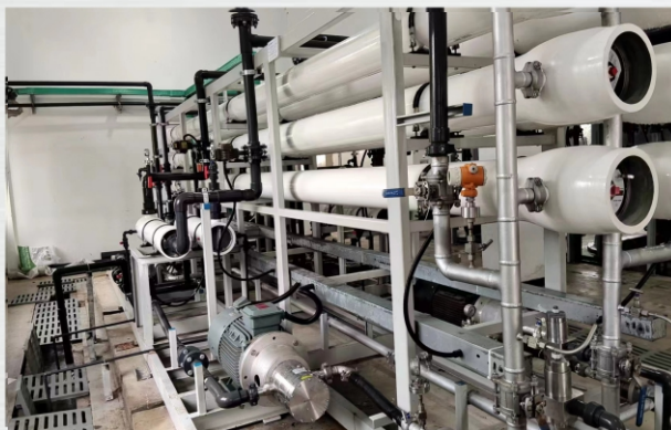
100t/d Seawater Desalination(DHP11 60Bar)
