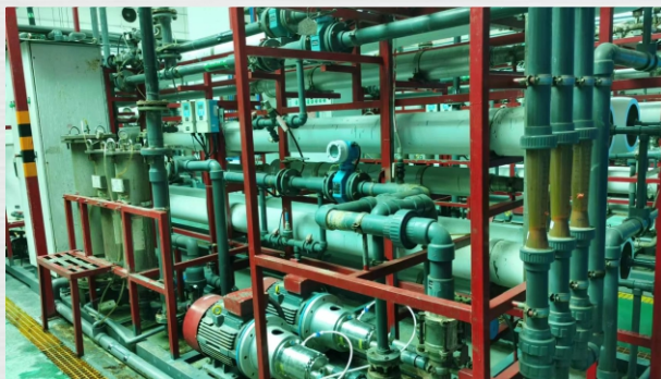
Landfill Leachate ZLD(DHP8.2 60Bar)
