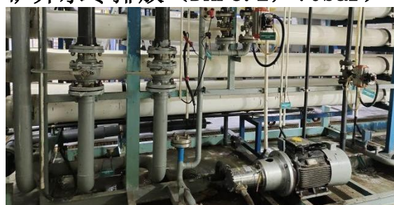
废水零排放 (DHP7.2, 80bar)
